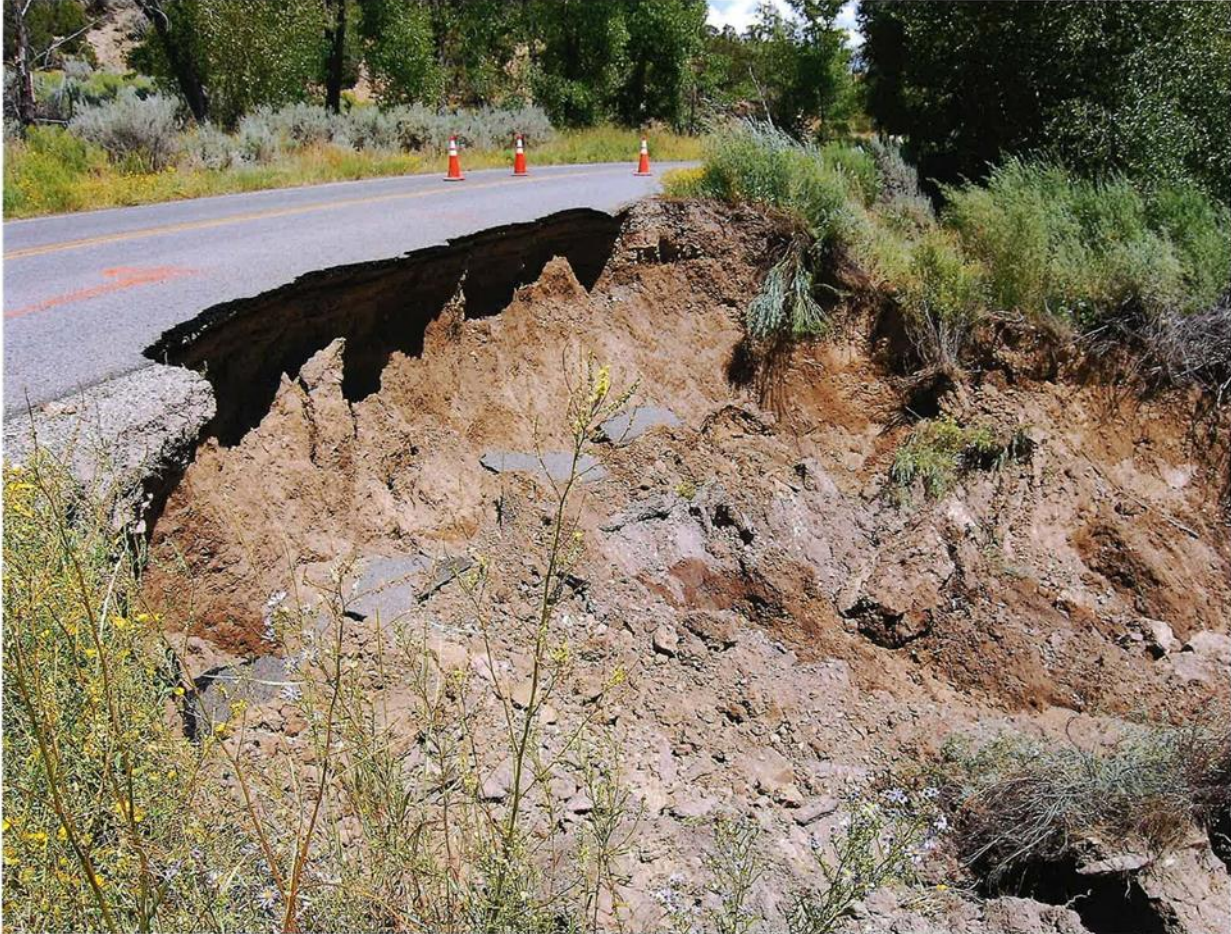
Erosion on County Road 237 near Harvey Gap in 2016
