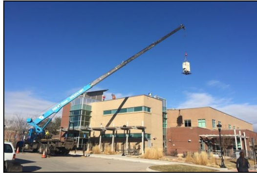
The Rifle camera, meteorological, and particulate monitoring equipment relocated to the roof of the Rifle Library.
