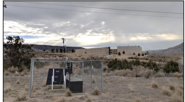
Downwind Sampler collects VOC samples when specific wind speed and wind direction conditions are present
